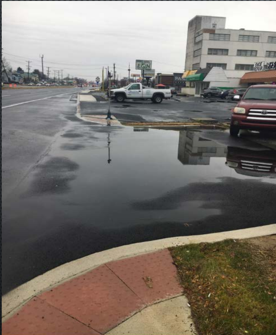
Kirkwood Highway PAR, Curb Ramp 12, December 10, 2019, Post Rain Event, 1:30pm
